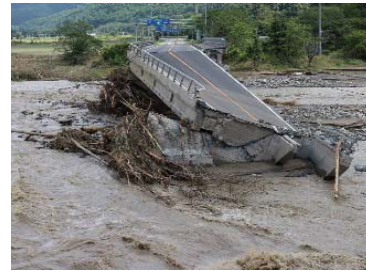
Photo 1: Road bridge of a national road damaged in a flood
