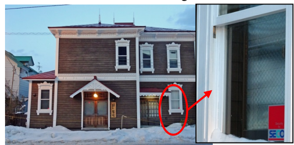
Photo 3. An example in which wire glass is used on the inside of an opening
