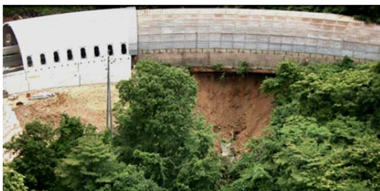
Photo 1: The entire view of Noboritani Snow Shelter and damaged section
