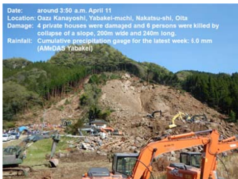
Photo 1: Collapse with no rainfall etc. at Nakatsu-shi, Oita
