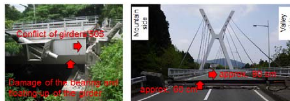
Fig.1: Main damage to the Kuwazuru Bridge
