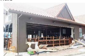
Outdoor fittings of stores Damage and collapse of large sashes
