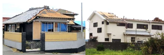
Scattering of roofing materials
