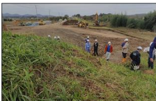
Photo 3 Collapse at 28.6 kp on the right bank of Naka River (Oct. 18)
