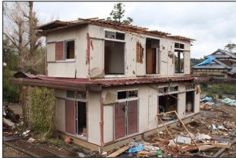
Photo 10 Damage to the roof, openings, etc. of a house (Oct. 15)
