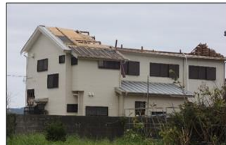
Photo 9 Scattering of the roof truss of a wooden house (Sep. 12)
