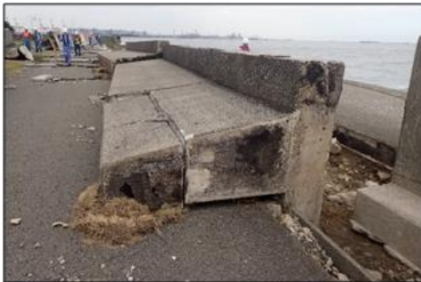
Photo 11 East side revetments in the Honmoku Futo district (Sep. 14)
