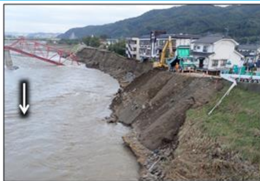
Photo 4 Levee collapse at 104 kp on the left bank of the Chikuma River Situation of damage (Oct. 15)
