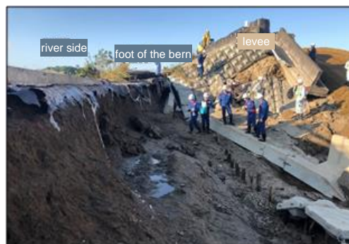
Photo 2 Collapse at 20.9 kp on the left bank of the Yoshida River in the Naruse River System (Oct. 16)
