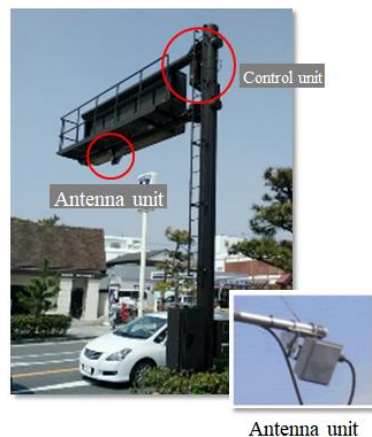
Example of ETC2.0 portable roadside unit installation
