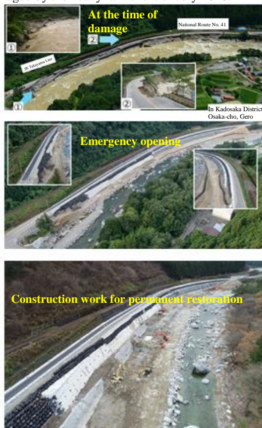
Fig. Photographs of damage to National Route 41 and the state of restoration
