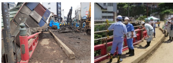
Aizomebashi damaged by sediment flow and on-site investigation
