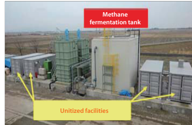
Picture External view of digestion and power generation facilities
