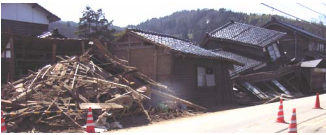
写真3 倒壊家屋が建ち並ぶ輪島市門前町館地区 Photo 3. Row of Toppled Homes in the Tachi District in Monzen-machi, Wajima City
