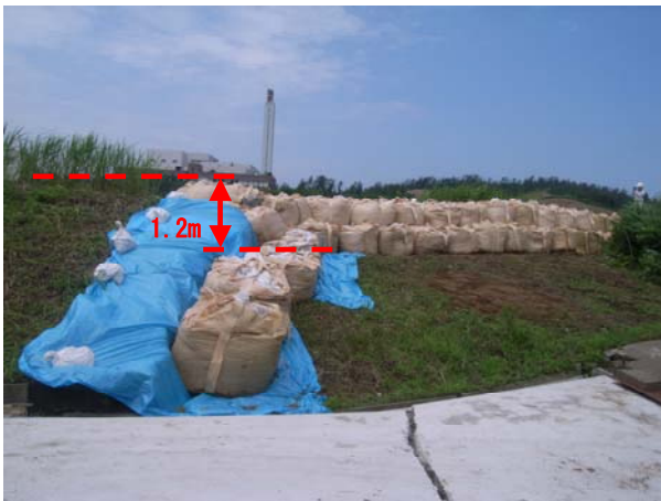
写真-2 鯖石川2kp付近左岸の横断亀裂を伴う沈下 Photo 2. Settlement caused by lateral cracking on the left bank near 2kp on the Sabaishi River
