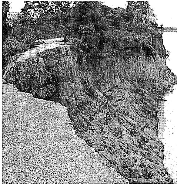
Road damage caused by riverbank erosion
