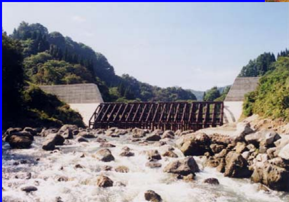
Masudama 2nd erosion control weir <transmissive> (Yamagata Pref.)
