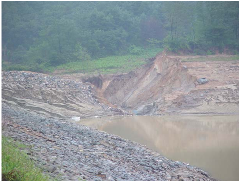
Figure 13. Dam collapse (Dongmak Reservoir; view from upstream to downstream)
