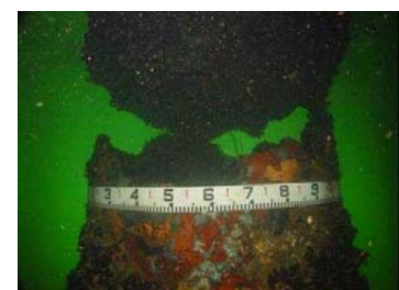
栈橋杭の破断
