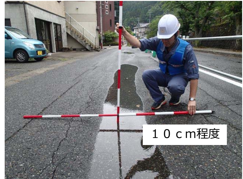
写真-17 陥没の深さ確認
