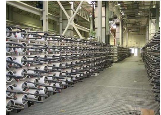
Reverse osmosis membrane purification facilities as part of the Groundwater Replenishment System (GWR System), Orange County, California, USA (in service since 2007)
