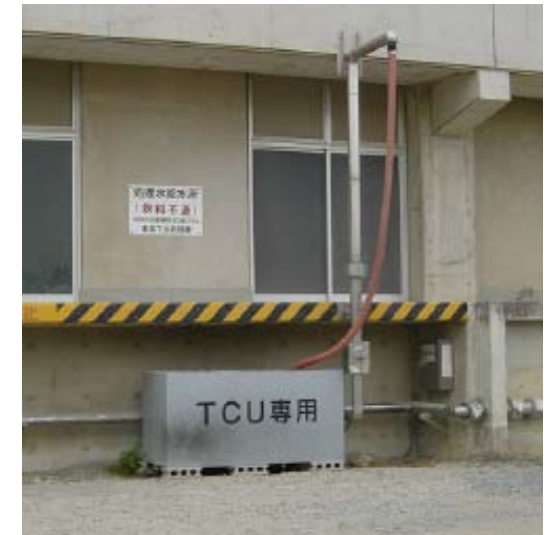
Filtered water outlet at the East Area Wastewater Reclamation Plant in Takamatsu City
