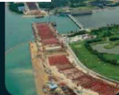
Marina Bay 滨海湾 Excavation and strutting work at Marina Bay 在滨海湾展开挖掘与支撑的工作
